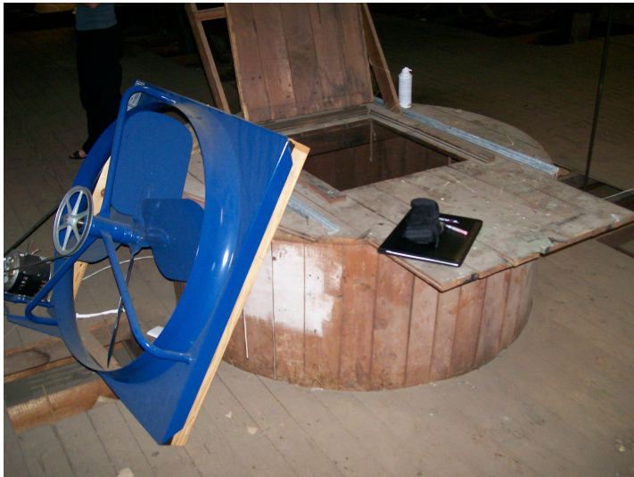
Vents above Chandeliers
